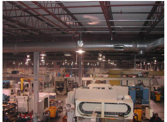
Figure 4: Soon after Tri Tool moved into their facility, complaints about the lighting system began.
