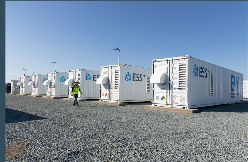
ESS Long-Duration Energy Storage
