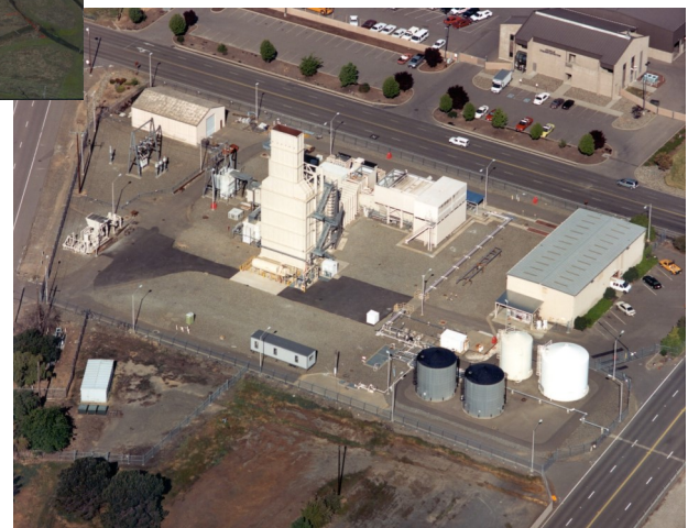
McClellan Power Plant
