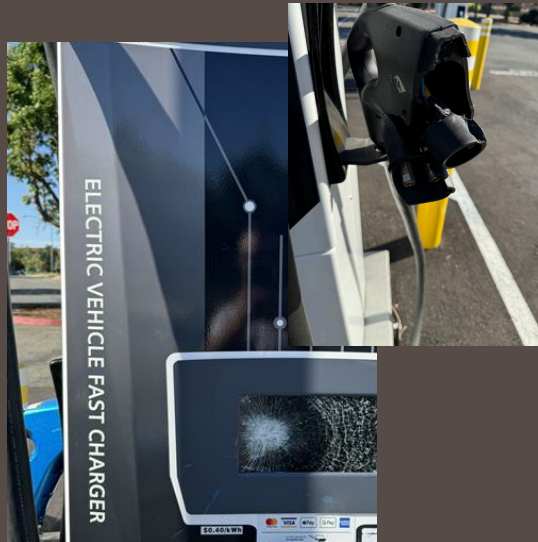
Charger Vandalism in Sacramento
