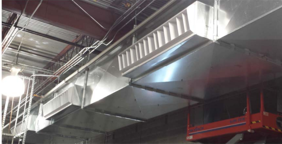
Figure 5: Large ducts for this manufacturing facility, bringing in much need fresh air. Note the system is balanced with an exhaust fan to not over pressurize the space.
