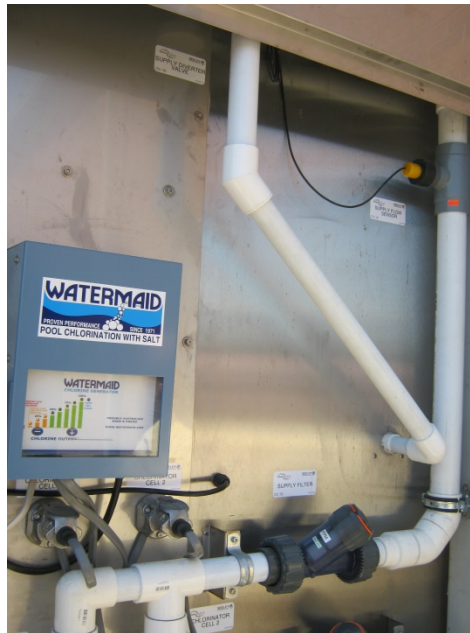
Figure 3: Chlorinator and plumbing for water circulation system, which reduces water consumption over continuous flow competitors but increases complexity.
