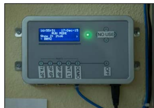
Figure 2: The fixtures in the patient rooms were controlled by a rather elaborate system that was intended for theatrical lighting applications.
