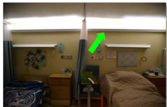
Figure 1: Because manufacturers did not offer tunable-white headboard fixtures in 2015, the team used linear LED fixtures inside of rain gutters to provide indirect lighting for the resident rooms.
