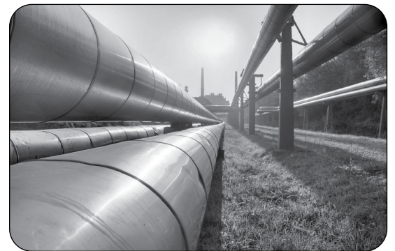
Pipelines are used to transport propane and natural gas to a processing facility.
