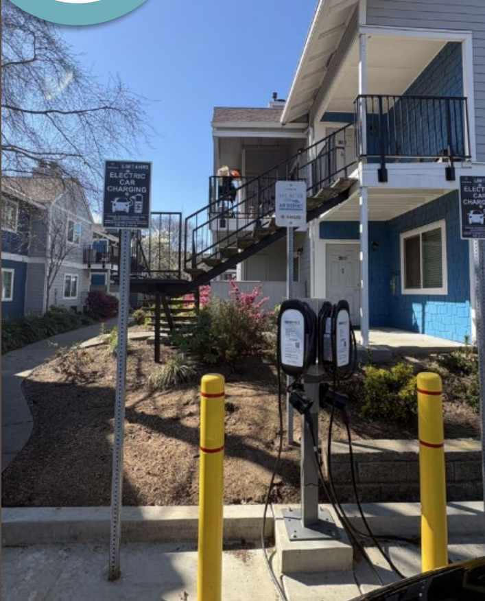
REACH 2.0 installation of 18 Level 2 chargers at Salishan multifamily community
