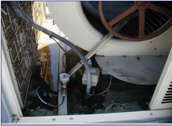
Evaporative cooler sump showing circulation pump and blow down water meter. Water meters were also installed on the make-up line to each unit.
