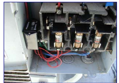
Hour meter on evaporative cooler main disconnect used to determine unit run times.
