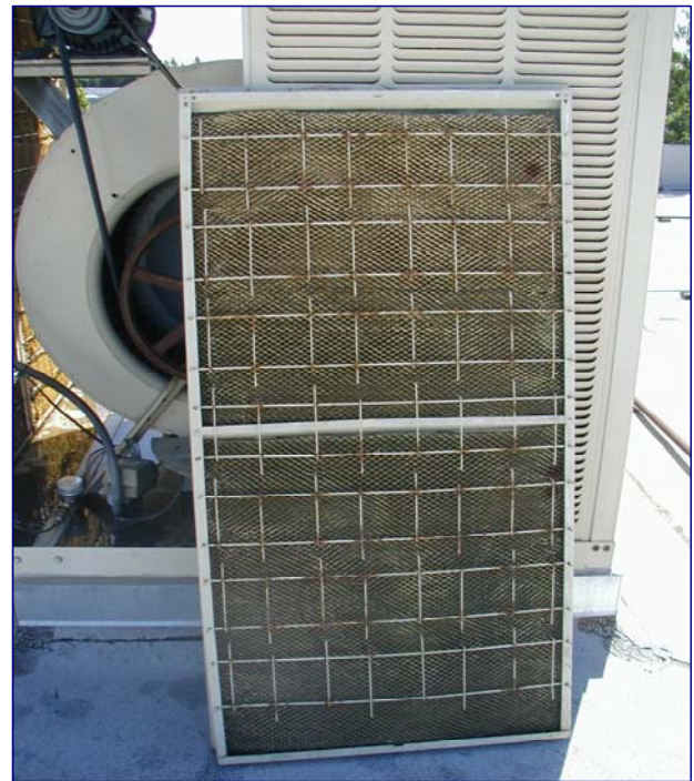
Two new evaporative pads in both the test and control unit were weighed before and after the study period to determine weight gain from salts of evaporation (scale)
