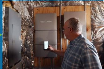
First customer grid-parallel deployment: Non-export with three Baltimore Gas & Electric (BG&E)
