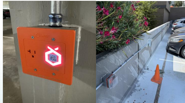
Smart outlets at Bridgeway Towers: 47 Level 1 (L1) "smart" chargers
