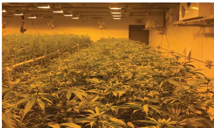
HPS fixtures installed in room 1.
