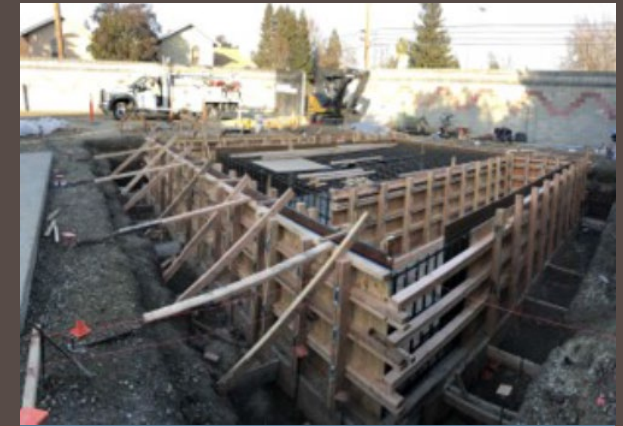
Distribution Sub Transformer Pad
