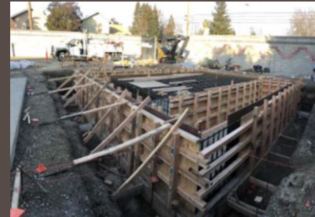
Distribution Sub Transformer Pad
