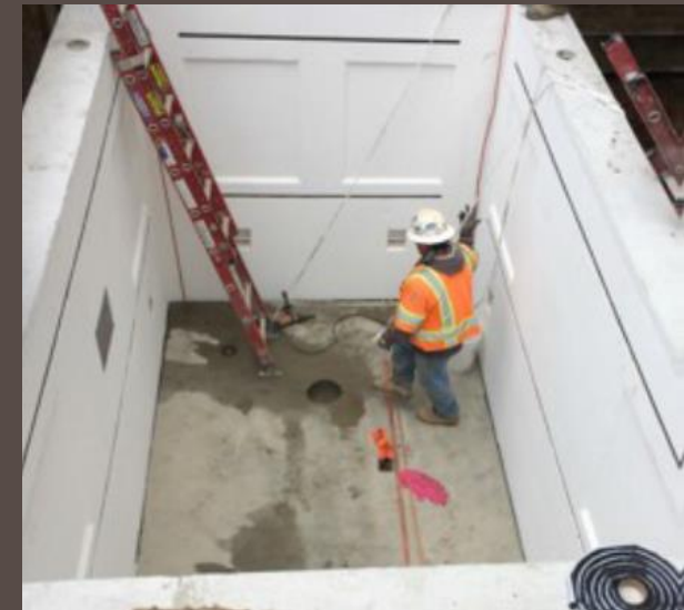
Distribution Sub 8 x 14' Cable Vault
