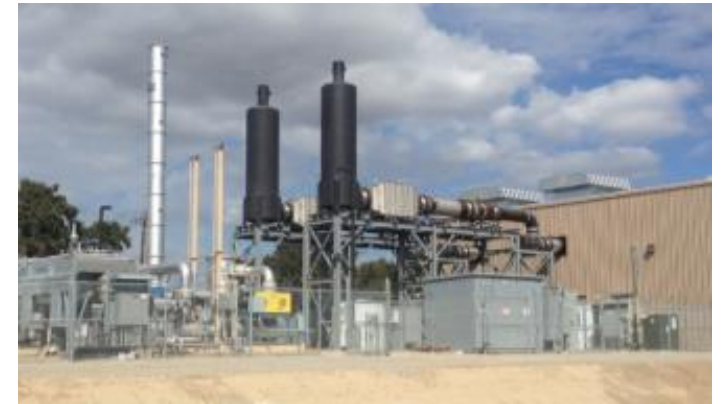
Landfill Gas To Electricity
