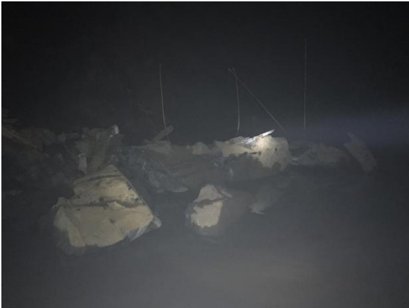
Bottom: Failed rock bolts in rockfall.
