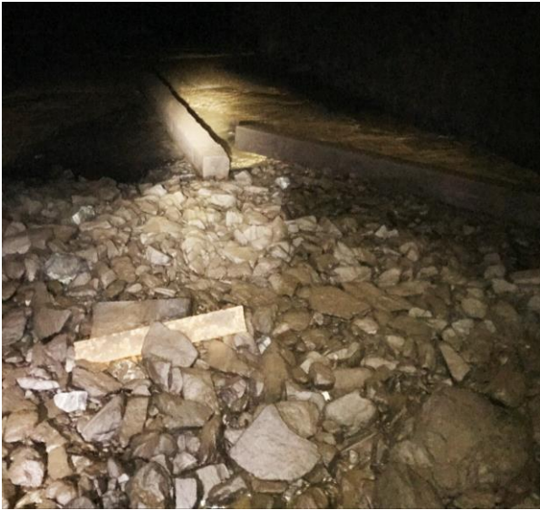
Top: Example of debris field discovered during tunnel inspection
