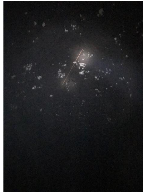
Failed rock bolt hanging from tunnel ceiling.
